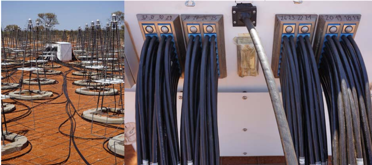
Figure 5: AAVS APIU and cable entry
