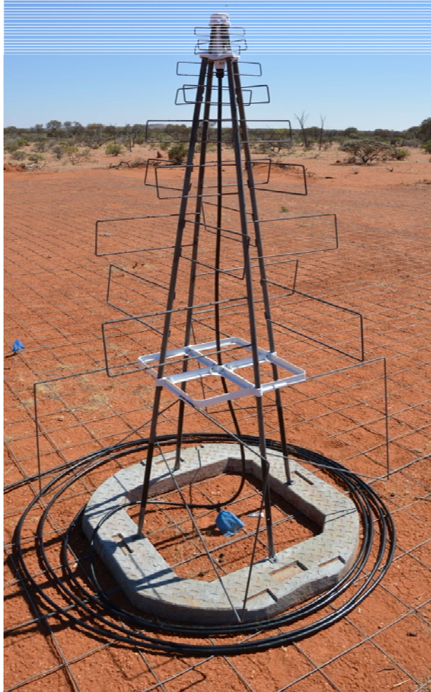
Figure 3: SKALA2 antenna installed in AAVS at the MRO
